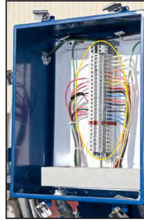
Figure 7 Terminal connections in burner junction box.
