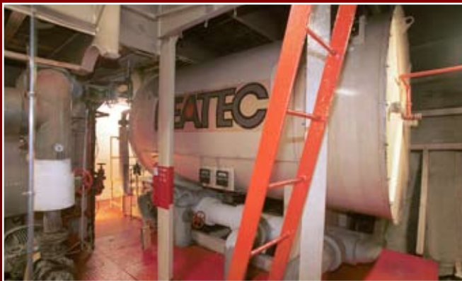
Heatec helical coil heater installed below deck on a barge. Heater is 10 years old.
