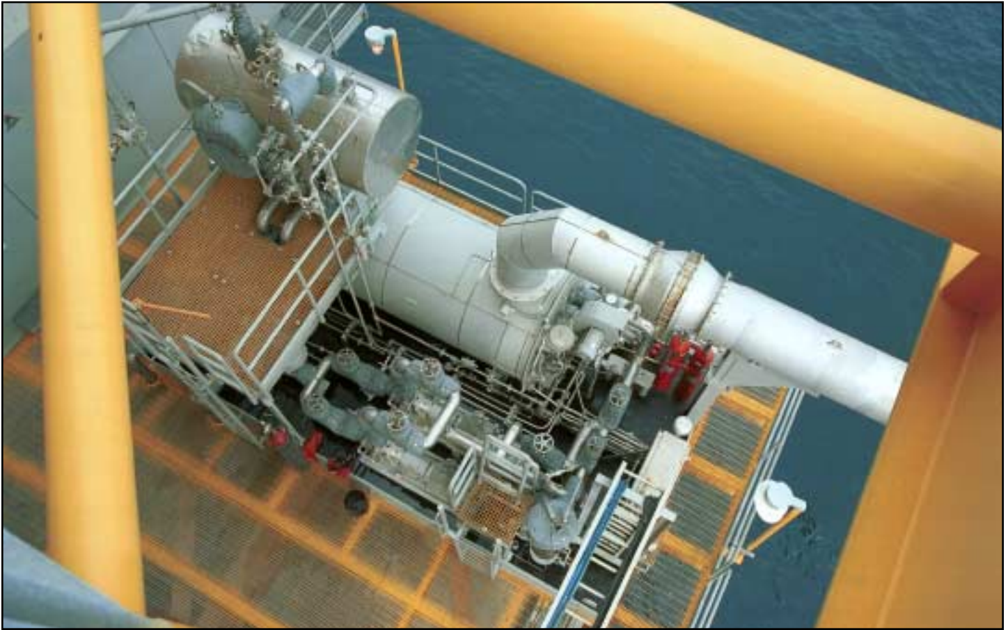
Heatec 5 million Btu/hour heater system on Hickory offshore platform
