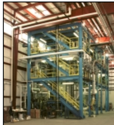
Krauss Maffei tray dryer installation
