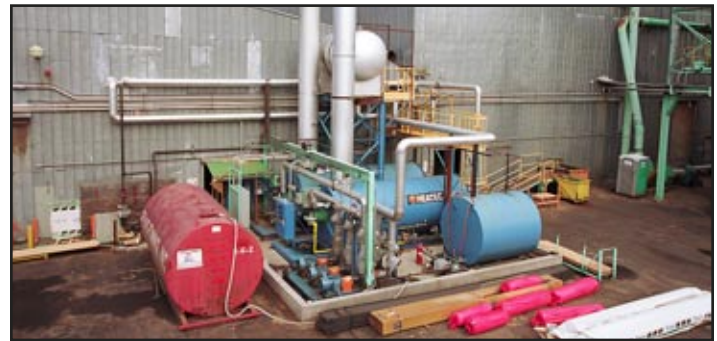
Two Heatec heaters at Eugene facility
