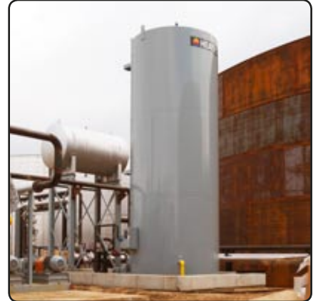
Vertical fuel tank, 20,000 gallon capacity.
