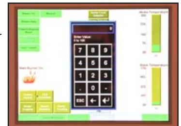
Another screen includes a key pad for changing set points. Simulated buttons allow other conditions to be selected for display. Bar graphs depict current temperatures and operating ranges.
