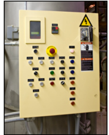
Control panel includes digital controller to set water temperature.
