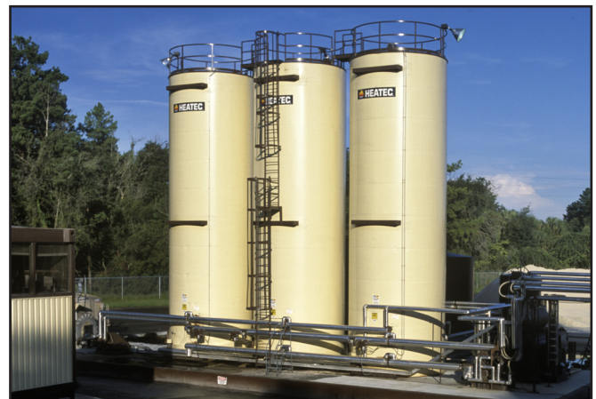
Figure 2. Heatec vertical asphalt tanks.
