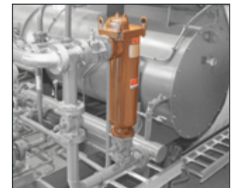
Sock filter (in color) and bypass valves installed in the thermal fluid piping of a heater.
