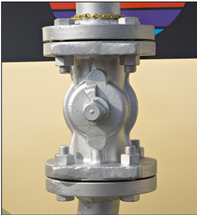
Figure 1. Typical flanged joints used in piping.
