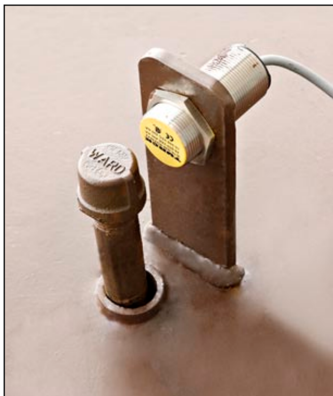
Figure 5. High-level proximity switch and float pipe protruding through sleeve in top of tank.
