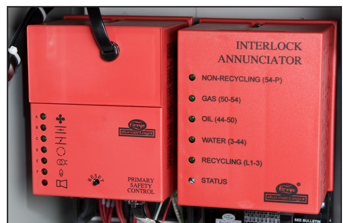
Figure 3. Burner control (left) and annunciator (right).
