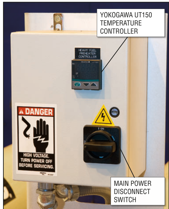
Figure 4. Control panel on HFP model preheater.
