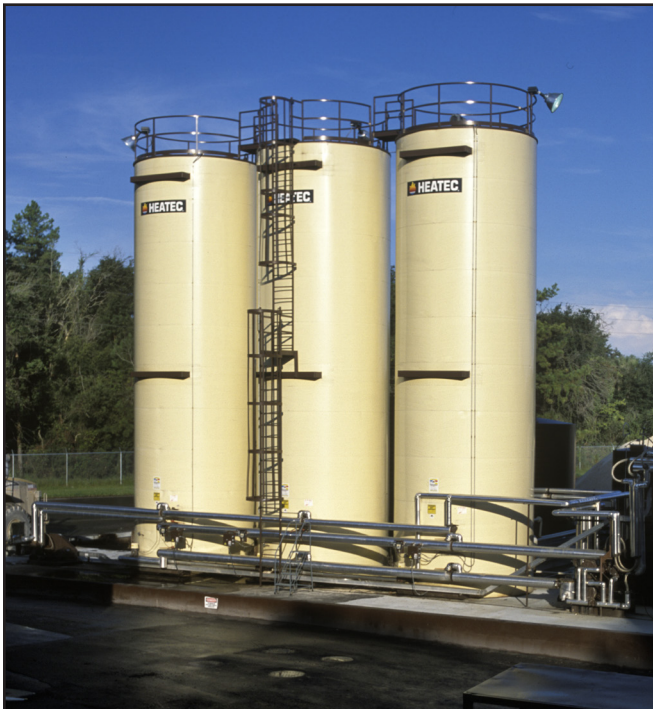
Figure 1. Heatec vertical asphalt tanks.
