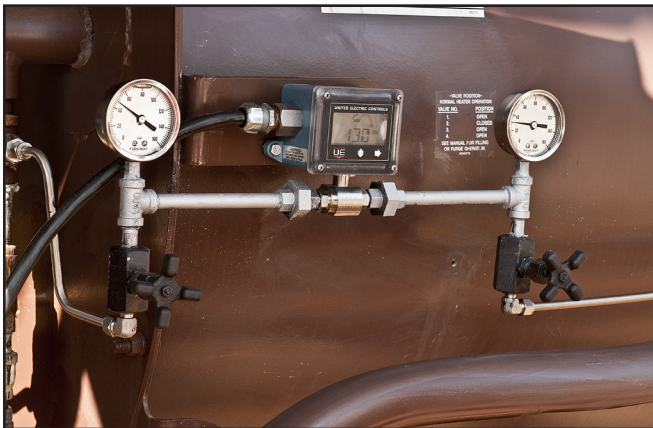
Figure 3. DP switch 4W3A01 installed on a Heatec heater.
